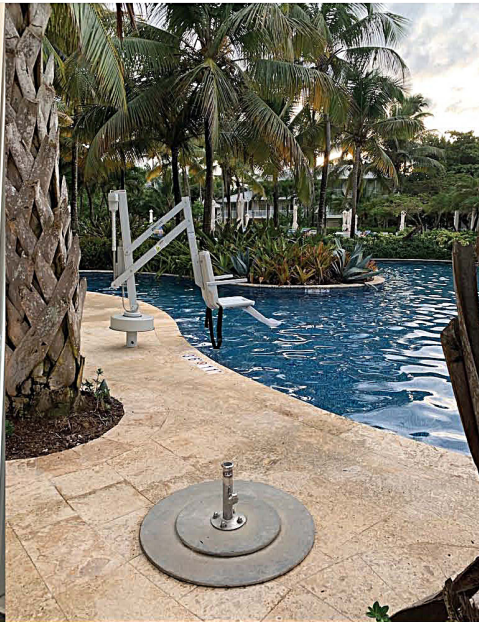
Pool lift, St. Regis Bahia Beach Resort, Puerto Rico.
